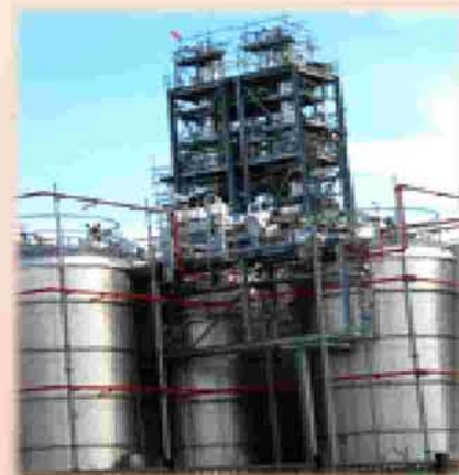
Solvent Recovery Plant
